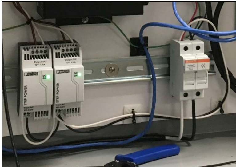
DC power supply units used to power the DCM6-L-CC mounted inside Frontier enclosure.
